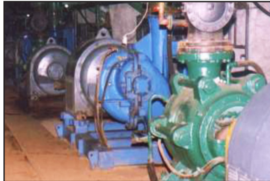
Bank of dewatering pumps
